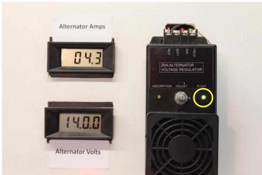
Float Phase: Green LED ON and battery at 14.00 V
